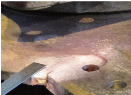
图 9 咬边缺陷处的疲劳裂纹 Fig. 9 Fatigue crack weld undercut clefect
